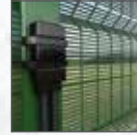
Fence Mounted IDS
